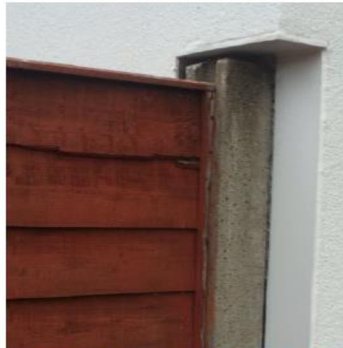
Figure 2 - Insulation not continuous behind fence post
